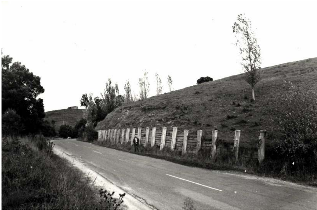
Figure 6.1 – Landslide no. 12, 1978. Stabilised by wooden retaining wall. Poplar trees have been planted to aid stabilization.
