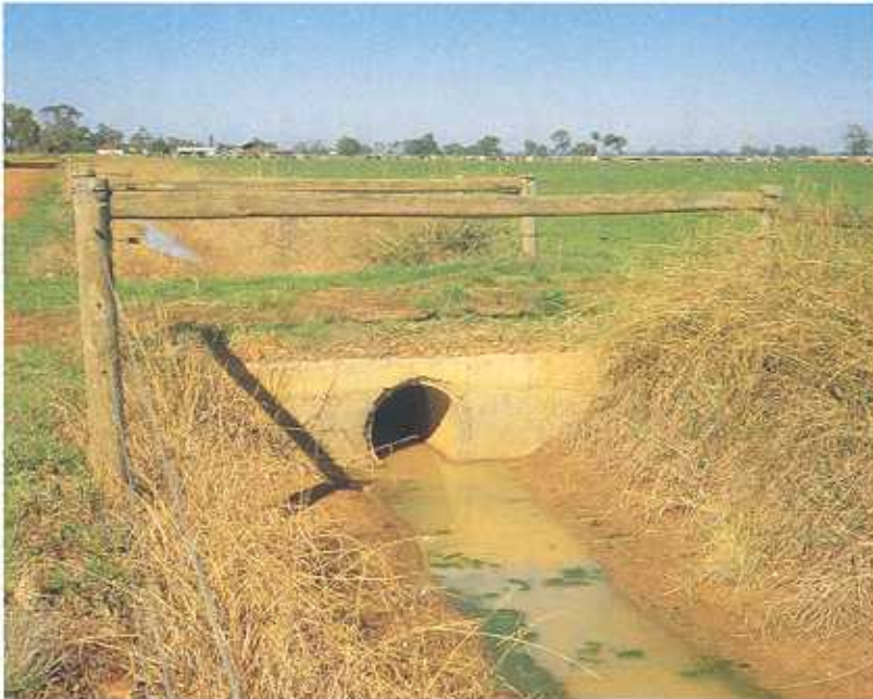
A channel crossing giving top access to the bay (see Diagram B overleaf)
