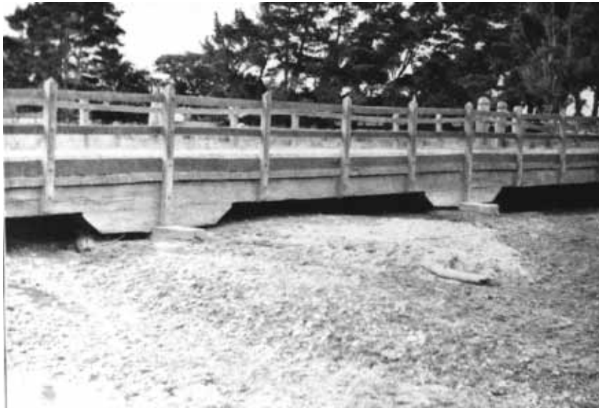
46. Bridge over Eaglehawk Creek on main Traralgon - Maffra road, near Glengarry. This has been so choked with debris from the scour shown in No. 26 that nearly all its capacity is gone, and the water in floodtime flow deep over the roadway, damaging it and holding up traffic.
