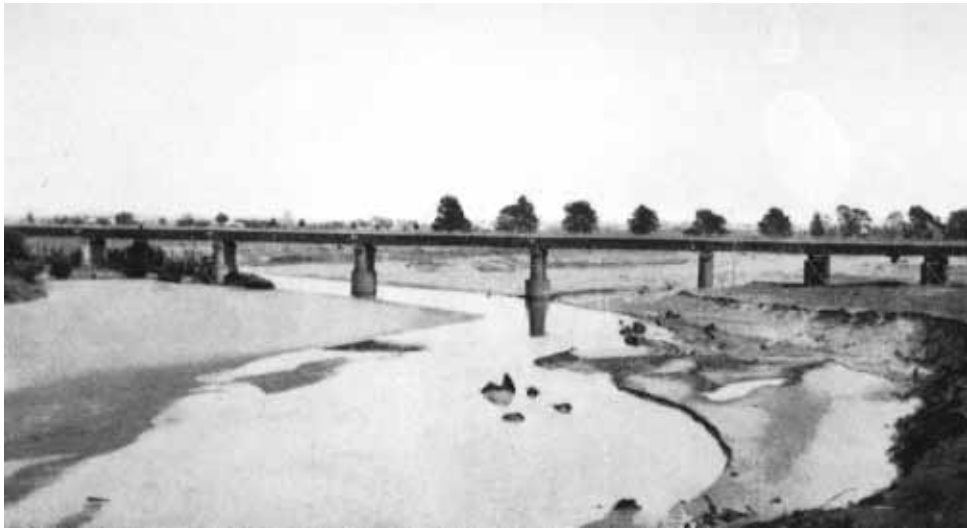
49. Railway bridge over Avon at Stratford. This has been lengthened by about 600 feet since 1886, and further extension will be necessary if further scour occurs.
