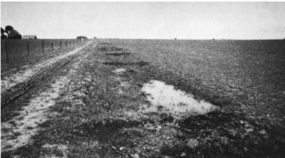
69. Small check dams of grass and manure constructed by land holder to check scour alongside road formation.
