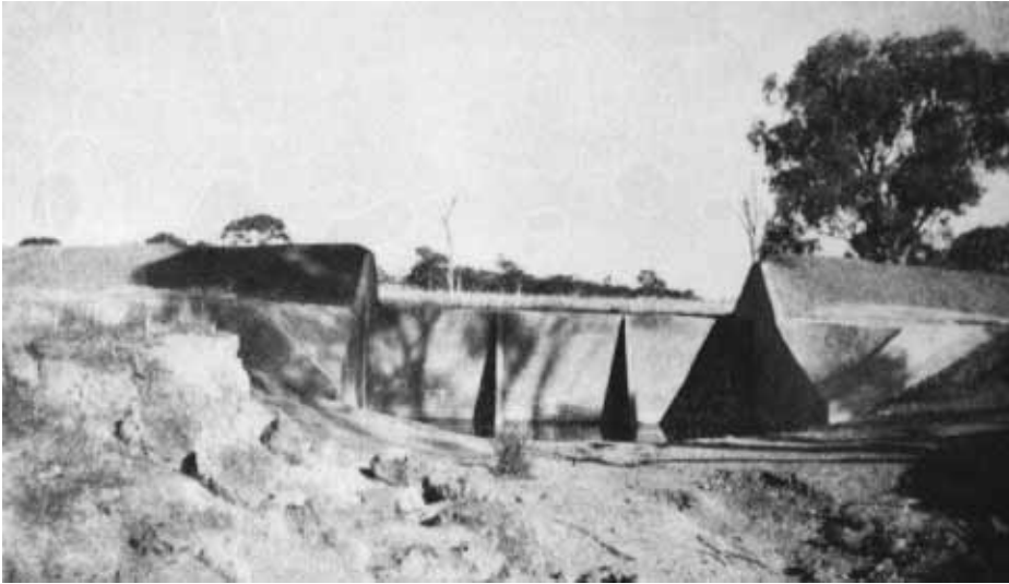
67. Concrete drop on the Sheep Pen Creek, at Caniambo. This is to check the extension of a branching scour, by concentrating all flow at a protected drop.
