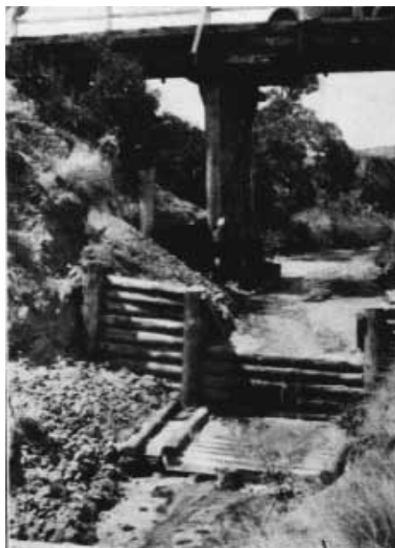
66. Small log dam constructed by Omeo Shire to protect road bridge over scouring gully.
