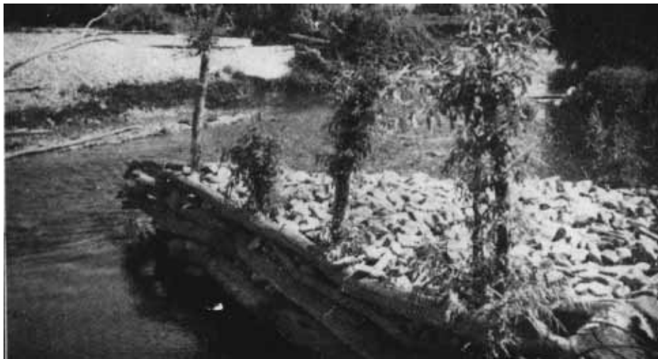
72. Up stream view of groyne installed by land holders on the Upper Tambo River.
