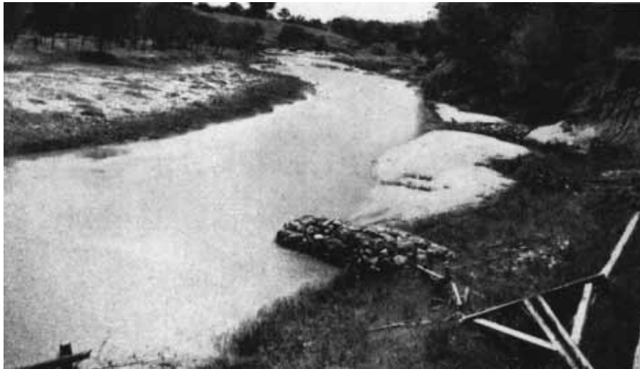
73. Small stone-wire mesh groynes in Yackandandah Creek to protect eroding bank. Note sand already deposited in twelve months.
