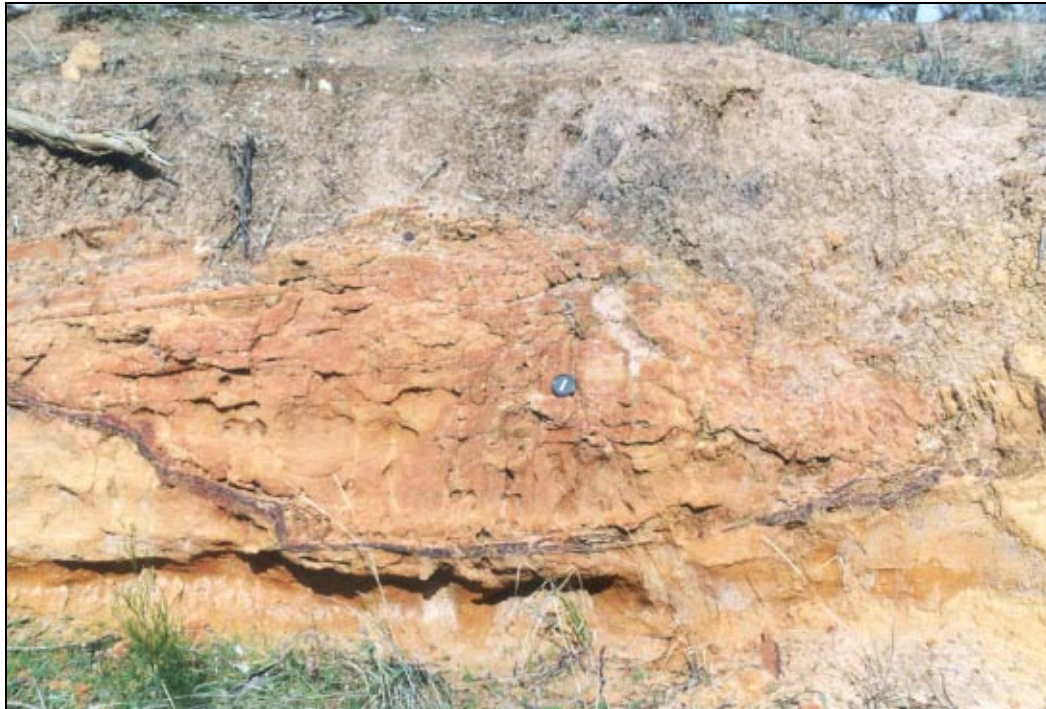
Plate 1 Road-cutting intersecting a Coarse Sand Rise landform unit displaying irregular ferruginised layers developed in the coarser sand beds which can inhibit deeper recharge (for scale, note lens cap near centre)
