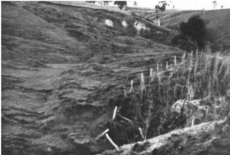
32. Landslides - Coleraine. Willows planted to bind the soil.
