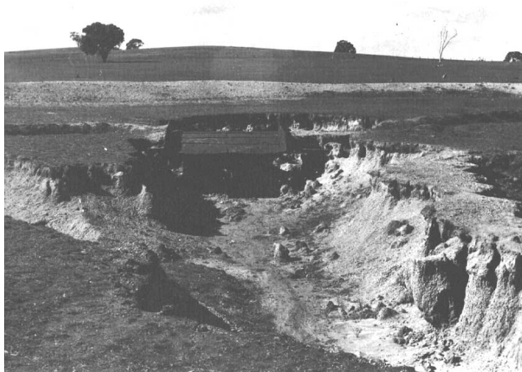
Plate 19. This verandah structure failed because it could not cope with A horizon sapping and deep tunnelling.
