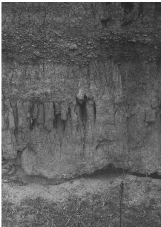
Plate 11. Tunnel erosion long cracks in burned soil (centre) and along Root-holes (top).
