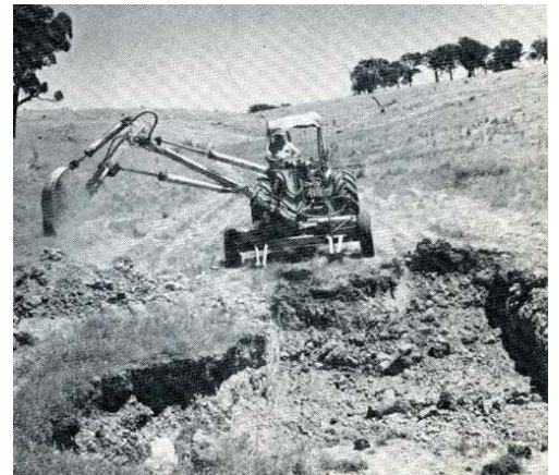
Building a grassed chute which will cope safely with run-off from the small catchment behind.
