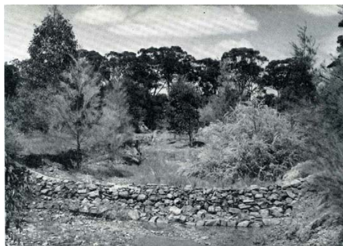
In many places in the Catchment loose stones were plentiful. They have been used here to build a silt trap in a large gully. Trees and other vegetation have been planted and are well established.
