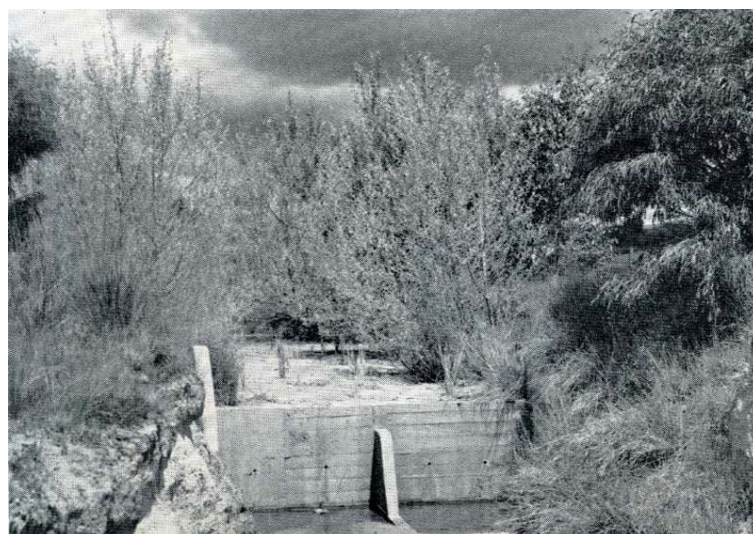
The same structure today; hundreds of cubic yards of silt have been trapped and vegetation holds it from further erosion.
