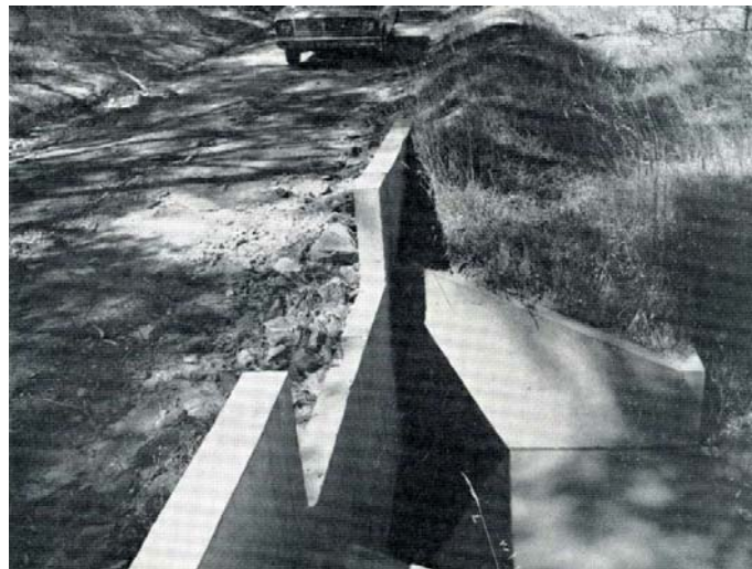
Here a gully had threatened the Shire road. This concrete structure is preventing any further erosion.
