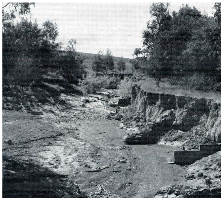
Note the different kinds of groynes (stone and timber) on the right-hand side of the gully which prevent further bank erosion. See also the trees which have been planted both in and around the gully.
