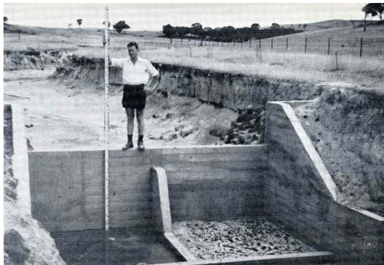
One of the hundreds of concrete silt traps that were built to prevent silt from reaching the reservoir.
