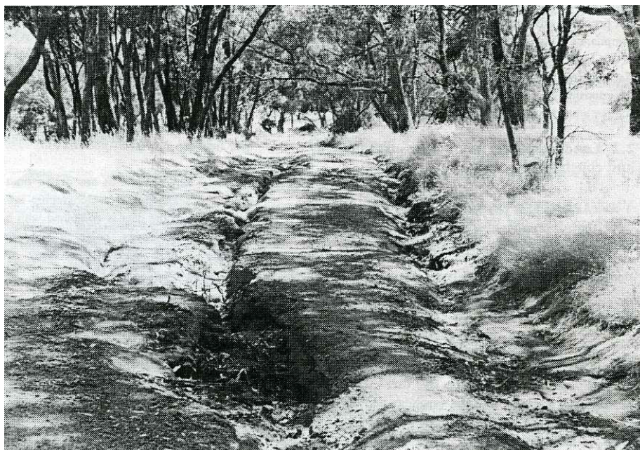
Figure 2.1 - Severe erosion of an unsealed road after heavy rains
