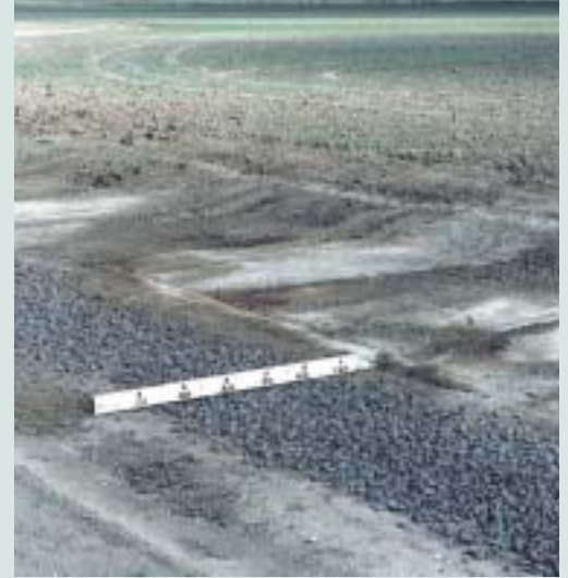
One of the finished underground drainage sections backfilled with 40mm clean gravel.
