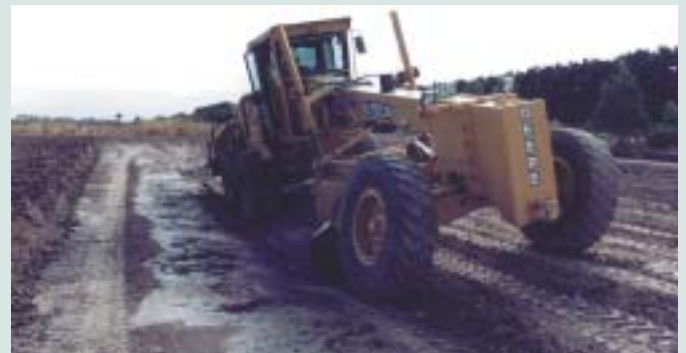
The road grader deepening the "V" drain by about 300mm ready to backfill with large crushed rock.
