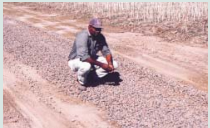
Gravel 40-50mm was placed over the pipe again using the grain truck. However this time a much larger chute had to be constructed for the truck to handle the larger diameter and angular gravel. Our photo shows Southern Farming Systems Soil Scientist, Renick Peries admiring the finished job.
