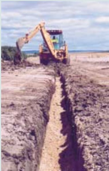
The backhoe digging the 450mm deep and 300mm wide trench. Note the spoil was removed while the backhoe was working and a gravel base added to the trench.
