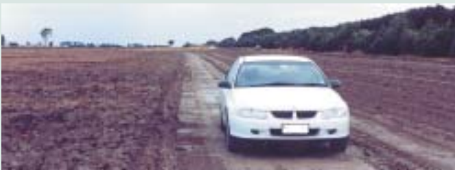
Using a dumpy level we determined the falls we had to play with and engaged a road grader to widen (25m) and heighten (650mm) the existing wide raised bed headland. With the road grader we placed a slope (1%) on the apron between the ends of the beds and the main drain. For our purposes, the main drain is "V" shaped and not flat as normally recommended.
