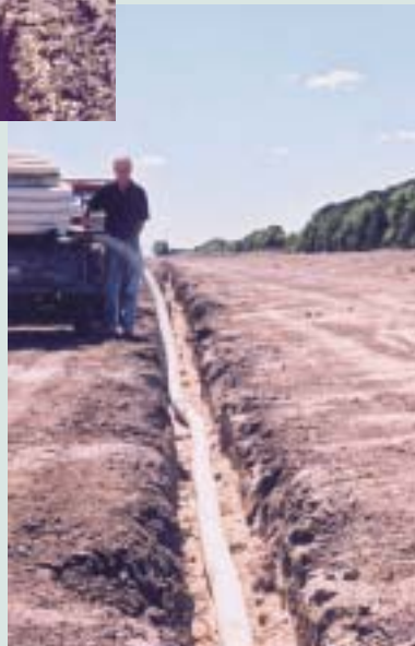
Pipe was fed off a reel directly into the trench. Note we have not used a fitter sock over the pipe. We will have to wait and see if that was a good idea. A small length of pipe with sock was installed to compare the difference over time.
