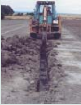
A backhoe digs a trench about 400mm deep ready to install the underground pipe for our second treatment. Although we used a 300mm wide bucket, probably only a 100mm wide trench would be required.
