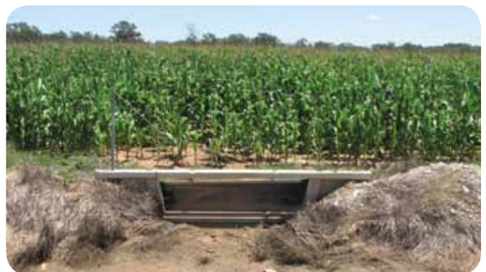
High flow Padman bay outlet
