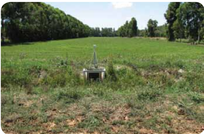
High flow piped Padman bay outlet
