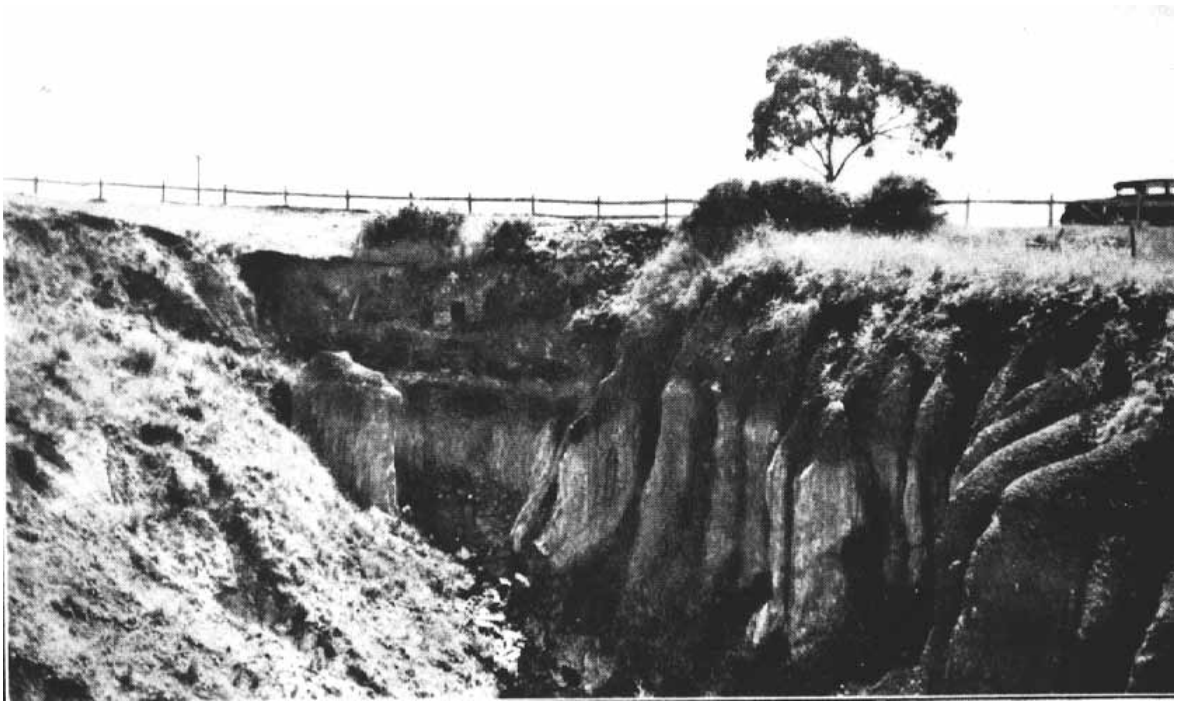
16. Scour below Bulla road, formed by small rectangular culvert through which storm water passes; may be seen in the left centre of the picture.
