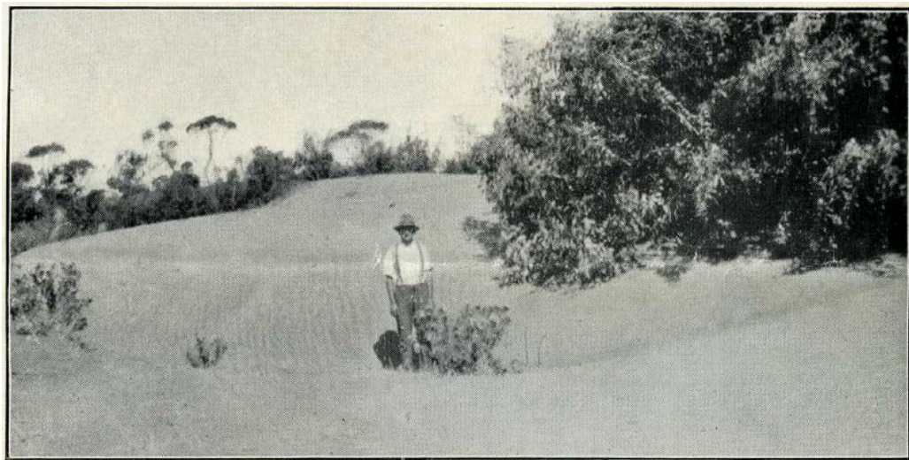
Tyrrell West Main Water Channel, near Sea Lake, completely blocked. 7,000 persons depend on this channel for their water supply.
