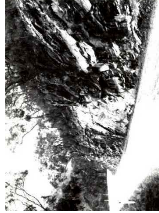
A typical roadside cutting within the steeply sloping Zumstein-Halls Gap area (Clk). Banks are usually broken and often unstable.
