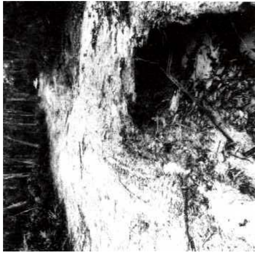
Gully occurring on sandy secondary roads of the gentle to moderate sloping terrain (Qrc) around the Wartook Reservoir.
