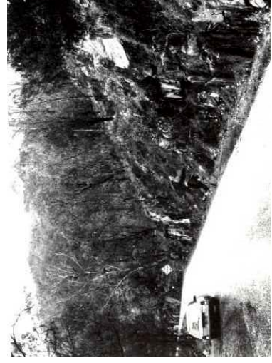
A typical steep sided road cutting in granite near Zumstein Park on the western side of the Grampians National Park.
