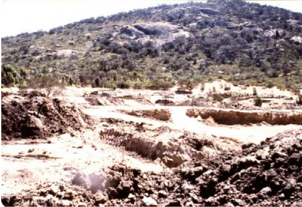
Plate 7 – Sand extraction operations have cleared and exposed large areas. Restoration will be both difficult and expensive.
