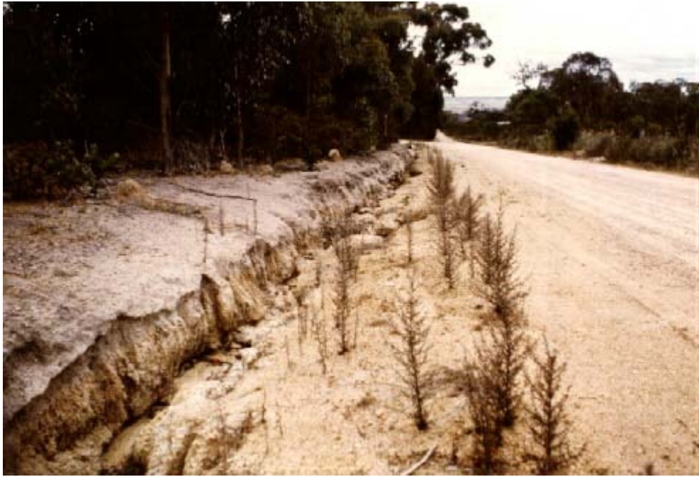
Plate 3 – Surface runoff from steeper areas can increase the erosion hazard
