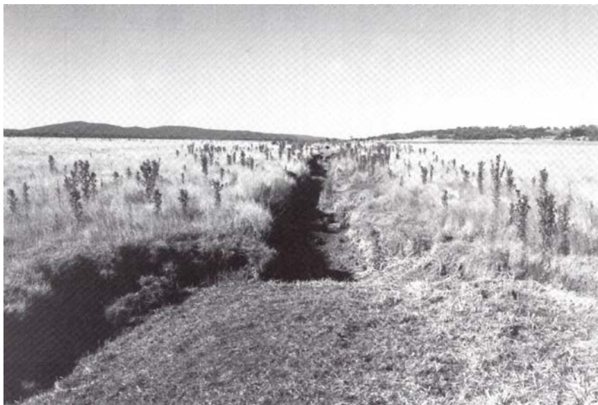
Increased run-off has scoured out this drainage ditch through a poorly drained area.
